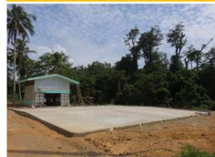
Solar dryer with warehouse in Brgy. Balubuan, Sirawai, Zamboanga del Norte with 858 estimated number of beneficiaries.
