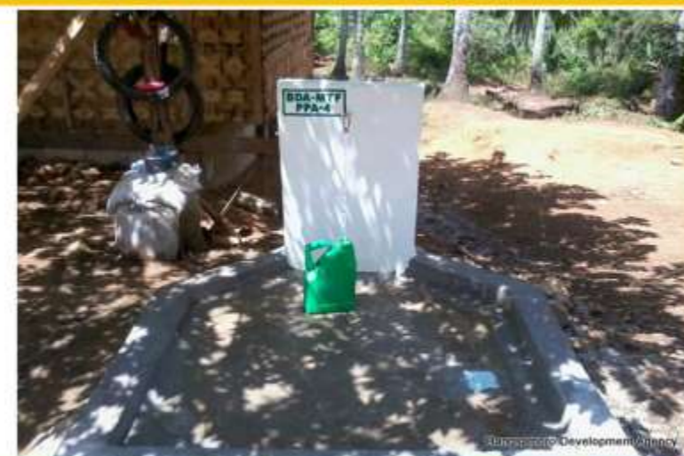
Water System Level II (Spring Development) in Brgy. Tubaon, Tarragona, Davao Oriental serving 664 beneficiaries
